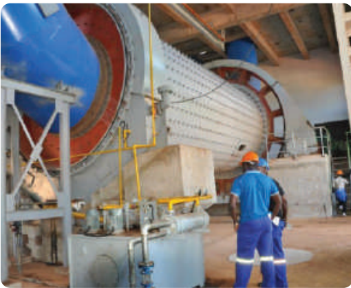
Fig 16.12 A production machine at the Bugarama cement factory
