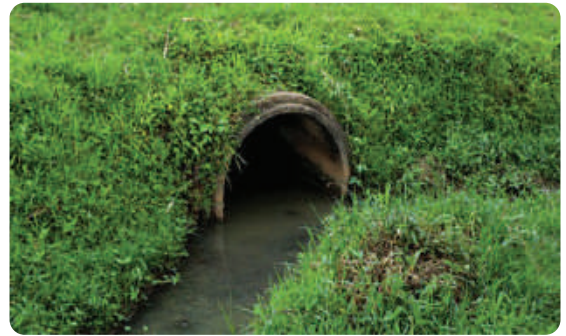
Fig 16.7 Improper disposal of waste from Kabuye Sugar Works
